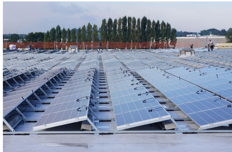
Solar panels at Mercury Marine's regional headquarters in Belgium produce nearly 460,000 kW. Photos courtesy of Brunswick.
